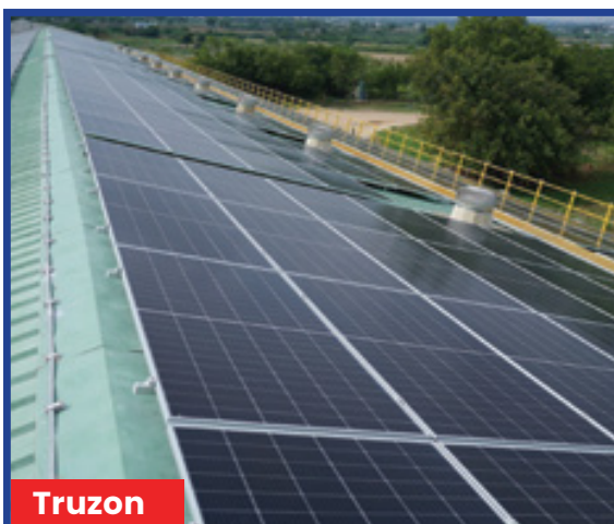
Improper Tilt Angle
